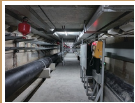
An underground pipe gallery in Guangming District, Shenzhen
