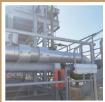
A Power Plant in Gibraltar
