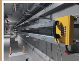
An underground pipe gallery in Binzhou City, Shandong Province
