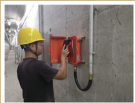
An underground pipe gallery on Honglian Road, Guangzhou
