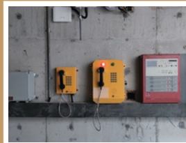
An underground pipe gallery in Dapeng District, Shenzhen
